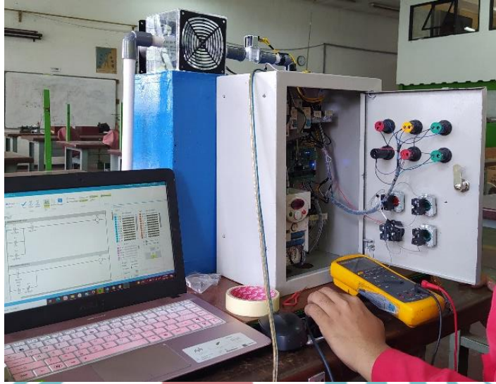
Gambar L. 24 Pengujian Panel Sistem Fan Coil Unit
