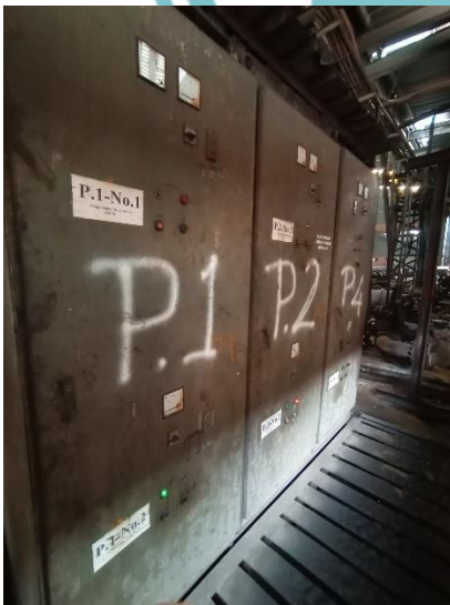
Panel Distribusi Pompa
