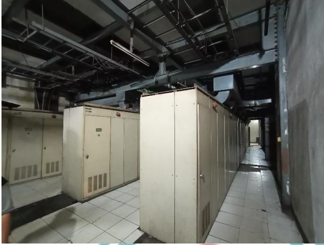
Ruang Panel Distribusi Substansi 2
