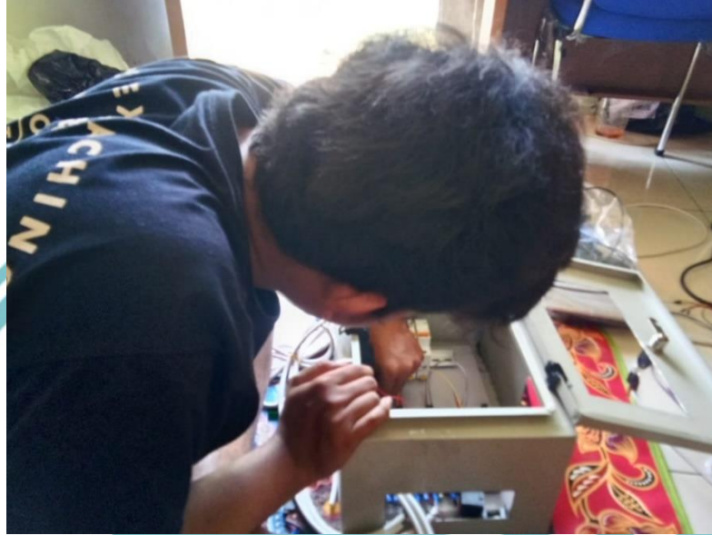
Lampiran 1. Proses Wiring Sistem Monitoring Panel Tegangan Rendah Berbasis IoT
