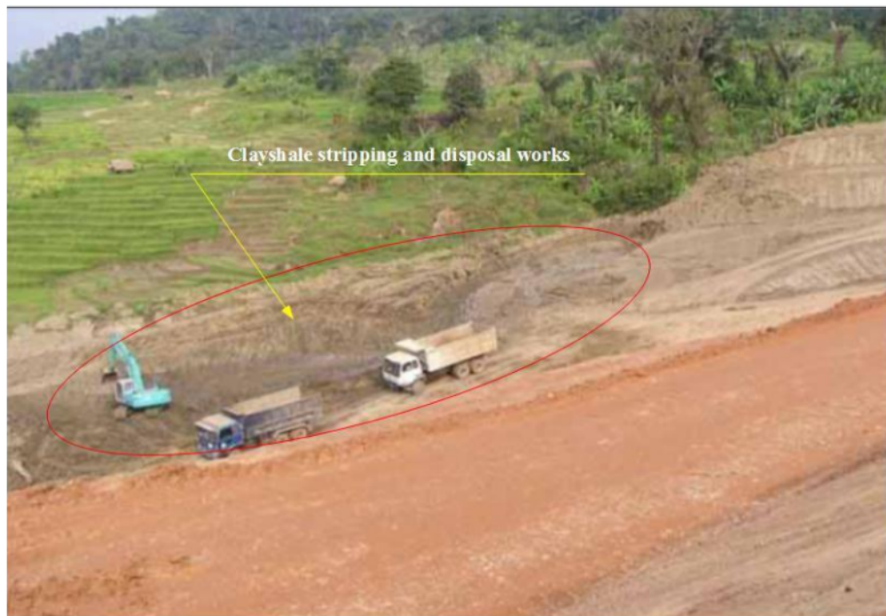
Figure 25. Stripping and disposal works for the upper layer (Jasa Marga (Persero), Tbk, 2003).
