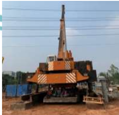
Gambar 4. 6 Kaki Alat Hidrolic Static Pile Driver (HSPD) Patah
