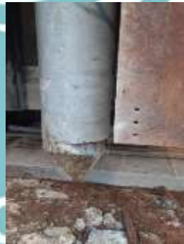
Gambar 4. 7 Spun Pile Patah
