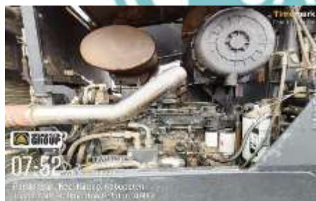
Failed Component (position at unit)
