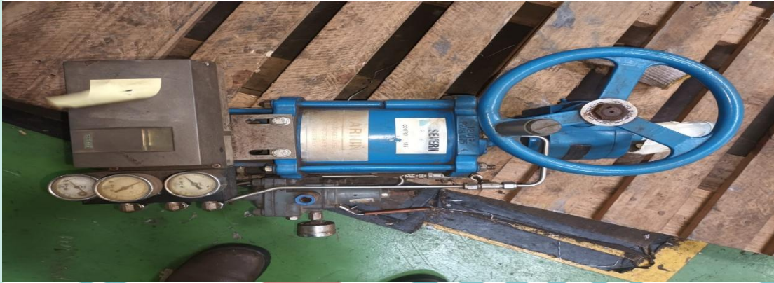
Lampiran 1. Dokumentasi Control Valve
