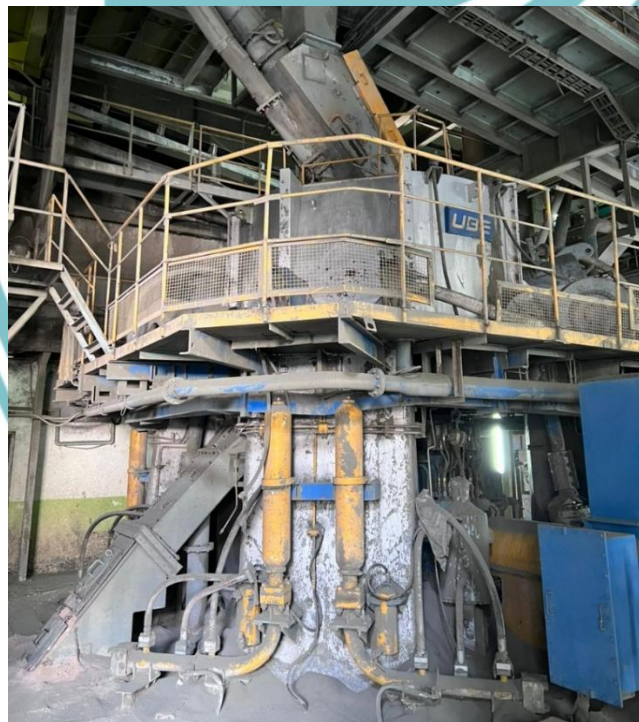
Gambar 2 2 Pre-Grinder Finish Mill Jalur 2
