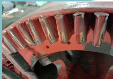
Gambar 4 6 Coil bar Rotor Insulation terbuka
