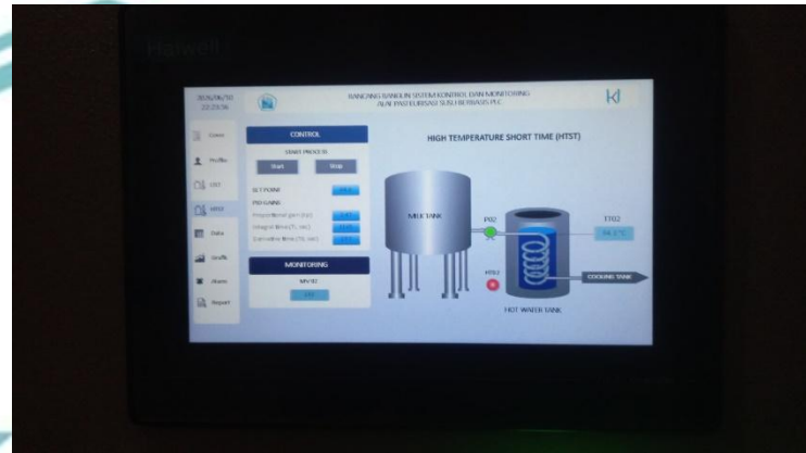
Pengujian Monitoring HMI
