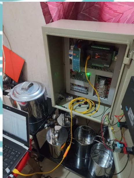
Running Program PLC
