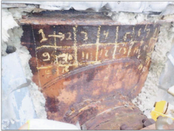
SHELL AREA MH-2 AREA 1
