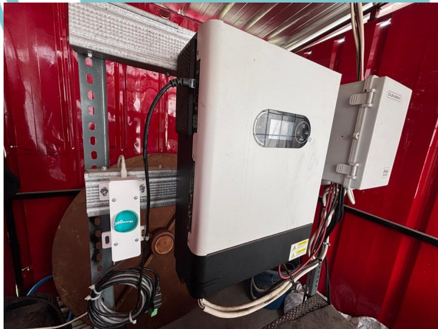
Lampiran 2. Tampak depan-samping inverter terpasang IoT gateway
