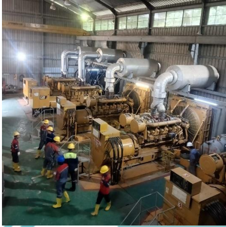
Power House PLTD
