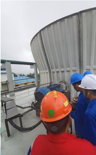
Pengambilan data vibrasi gearbox cooling tower
