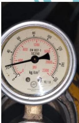
Pengecekan N2 Gas Accumulator
