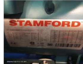
NAME PLATE GENERATOR
