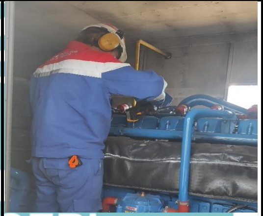
Pengecekan Suhu Exhaust Manifold
