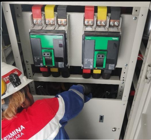
Pengukuran Arus Panel Feeder Comp. 1
