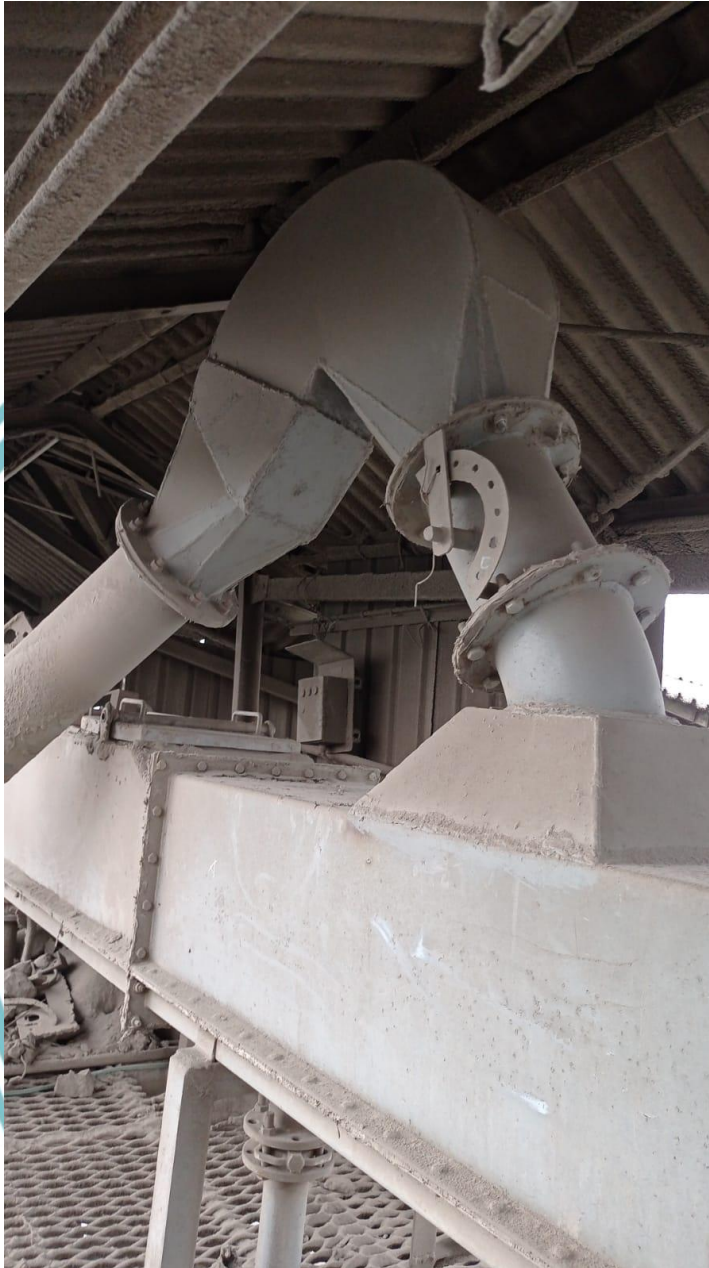
Lampiran Hisapan Ducting Tampak dekat
