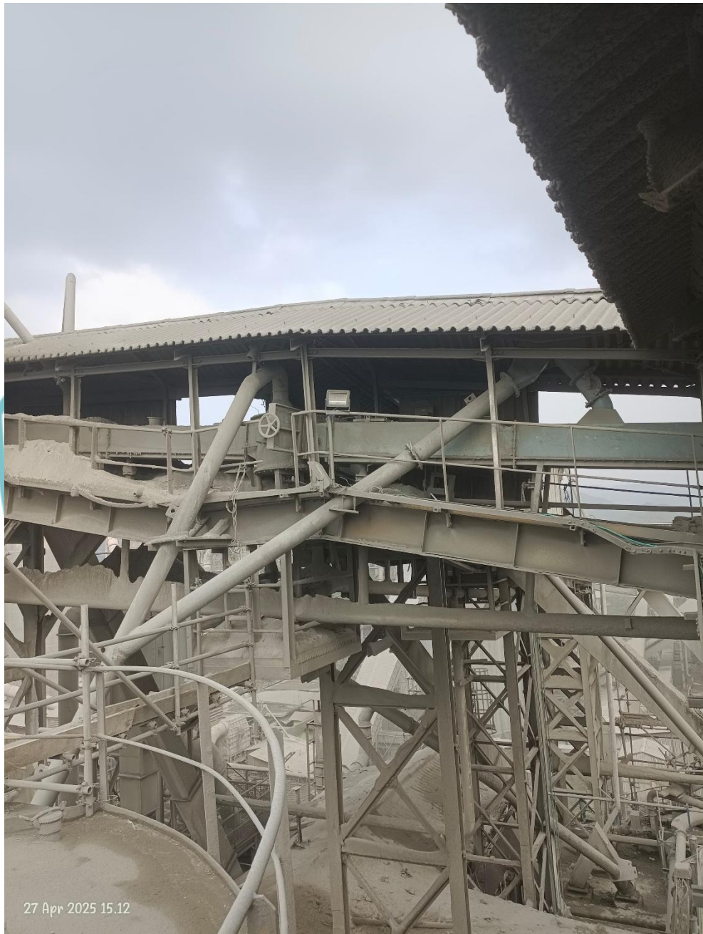
Lampiran Hisapan Ducting Tampak Jauh
