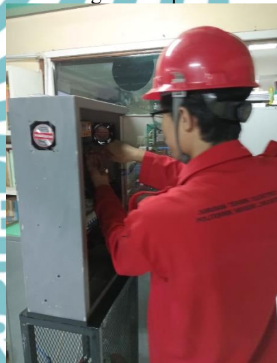
Proses Maintenance Sistem UPS
