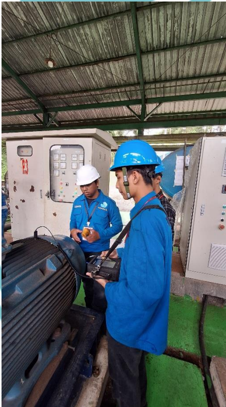
10. Running operation test ACWP dan CCWP unit 4
