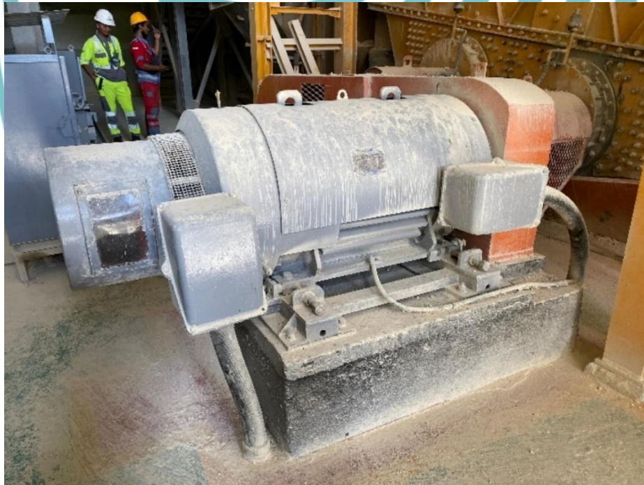
Gambar 1. 6 Slip Ring Motor Vibrating Screen 212-VS1
