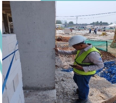
(Monitoring defect kolom)
