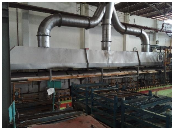
Sumber: Dokumen PT. GS BATTERY.
