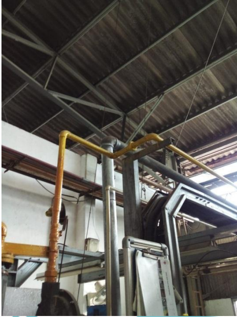
Sumber: Dokumen PT. GS BATTERY.
