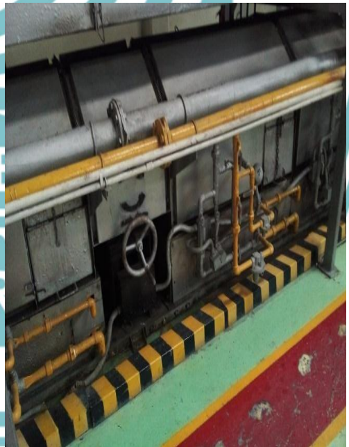
Sumber: Dokumen PT. GS BATTERY.
