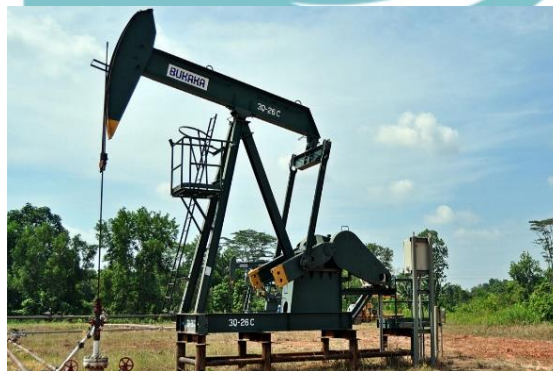
Gambar 3. 1 Struktur Pumping Unit
