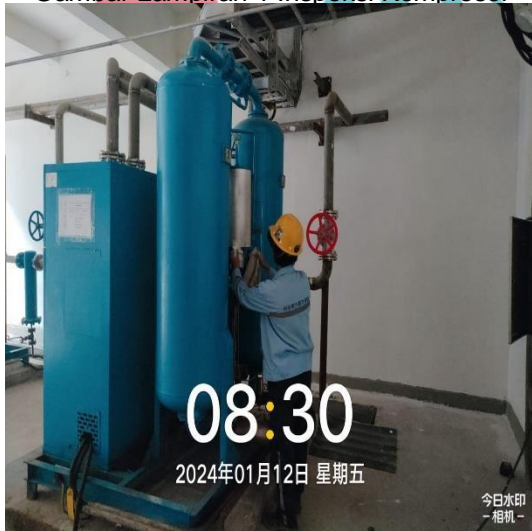
Gambar Lampiran 2 Cleaning Area Kompresor
