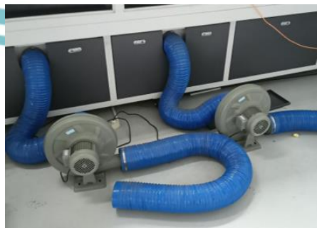
Gambar 3.6 Exhaust Fan Laser Cutting Machine VK-3015
