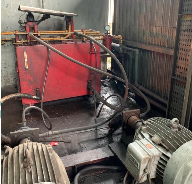
Lampiran 9 Pompa Hidrolik Furnace
