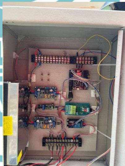
Panel Kontrol dan Monitoring
