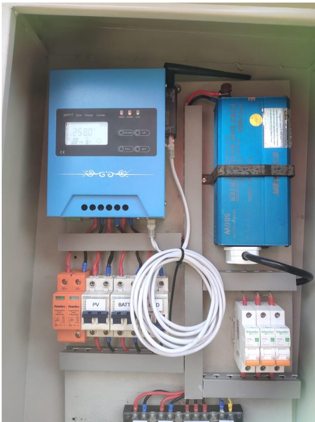
Gambar Penampakan box panel
