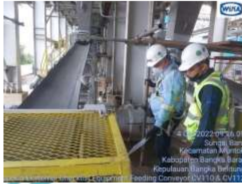
Inspeksi instalasi ceklis equipment
