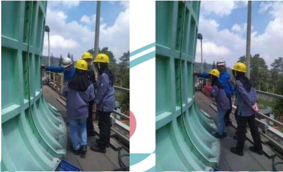
Gambar Pengecekan Fan Cooling Tower
