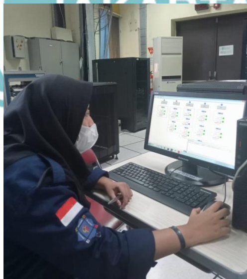
Gambar 3. 2 Pengecekan pada Remote Control Monitoring System
