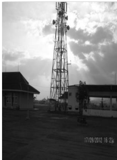
Gambar 2. 1 Self - Supporting Tower
