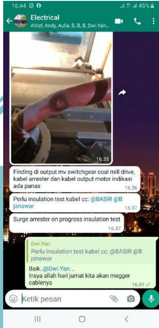
Gambar 1. 2 Isolasi cable output terbakar didalam cable compartment
