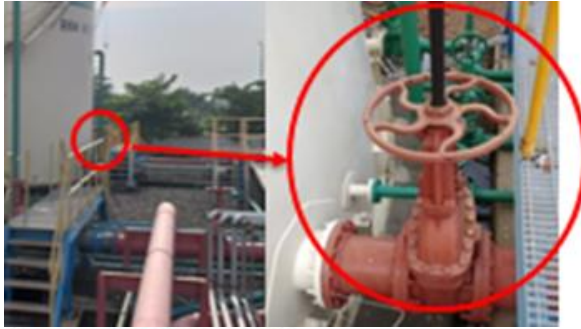
Gambar Valve return line fire fighting di RAW Tank 1
