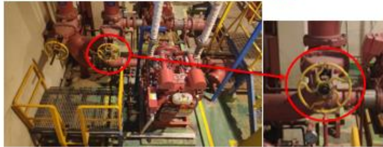
Gambar manual valve discharge to sea 9oSGA04oAA0o1
