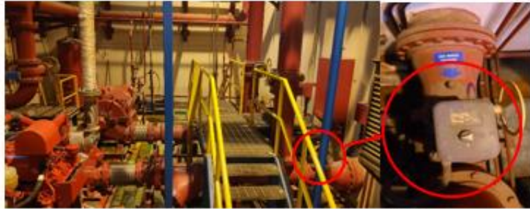
Gambar valve suction sea water 90SGA010AA002
