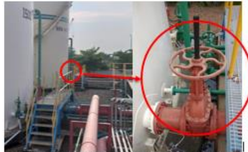
Gambar valve suction line firefighting pada RAW Tank 2
