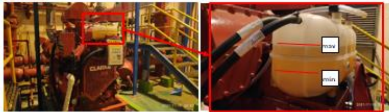
Gambar level water coolant diesel fire fighting pump
