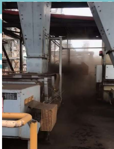
Gambar 1. 1 Pencemaran akibat debu batubara saat transfer material
