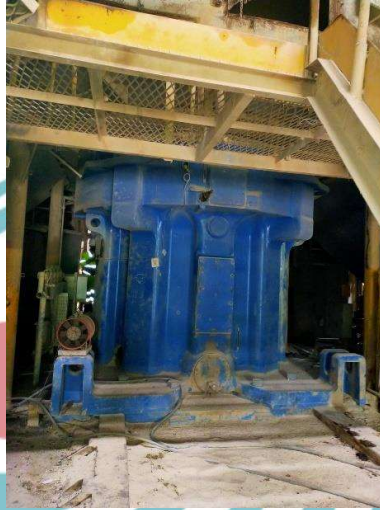
Gambar 1. 2 Reducer Roller Mill 362-RM1
