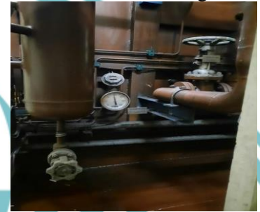
Temperatur oil tank
