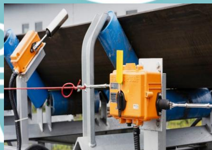
Gambar 2. 27 Pull Wire Switch
