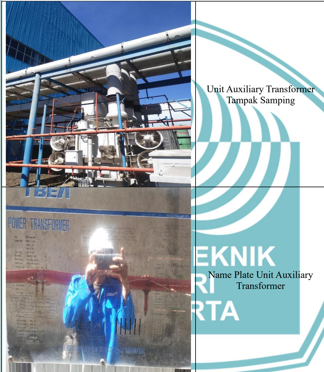
Lampiran 1. Foto Unit Auxiliary Transformer
