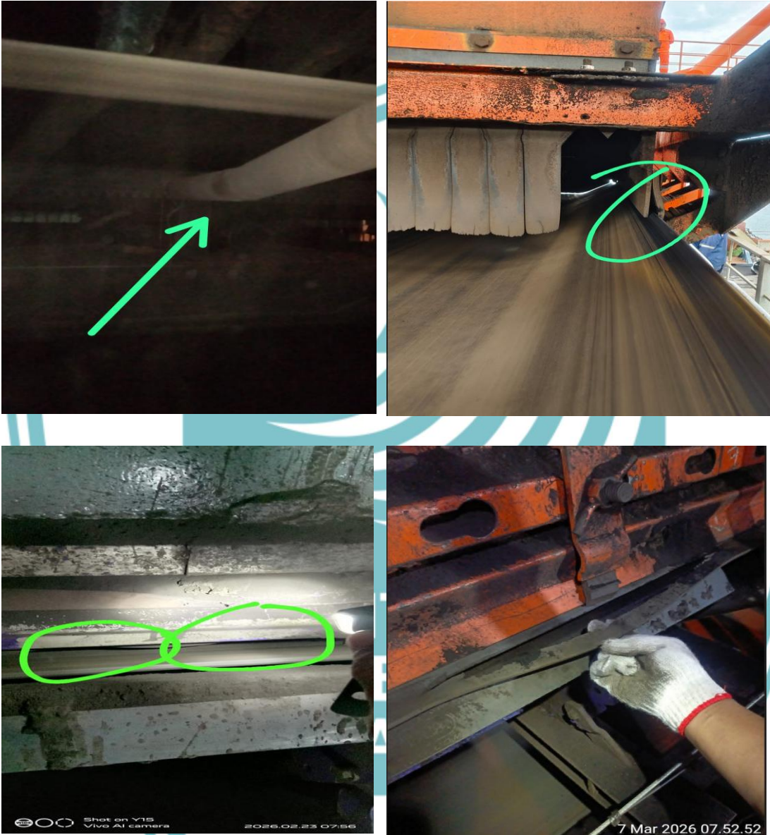
Lampiran 2 Gambar Kerusakan Belt Conveyor
