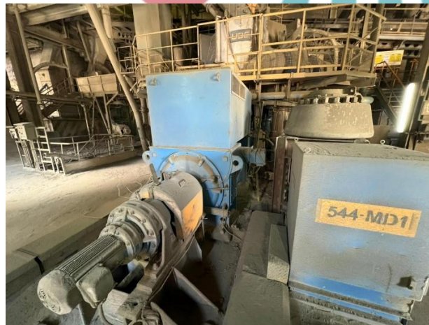
Gambar 1 1 Lokasi Aktual Main Drive Motor Pre-Grinder Finish Mill 544 – MD1
