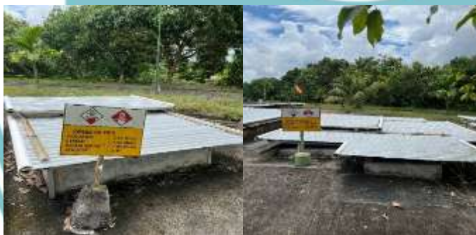
Gambar 1.1 Fasilitas Oil Pit & Oil Catcher di TPS Area IX
