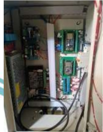
Gambar L-2 2. Hasil Wiring Panel
