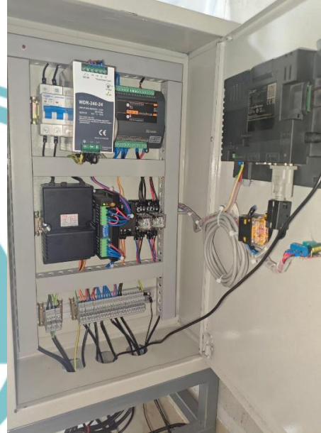
Wiring Panel Kontrol
