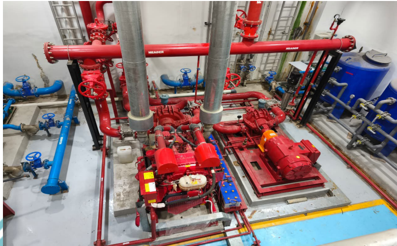
gambar 1.1 Hydrant pump Sentrifugal di Gedung Mandiri Financial Center
