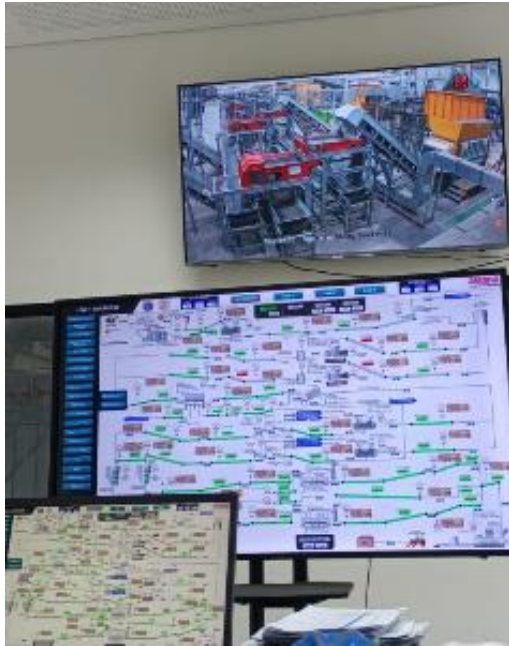
Operation Room (Scada)
