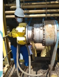
Gambar 12 PM Submerged Scraper Conveyor
