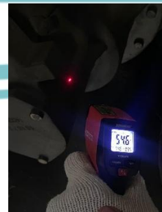
Gambar 8 Pengukuran Suhu Screw Compressor
