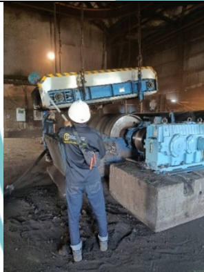
Gambar 5.9 Cleaning Knife Valve Separator BC
