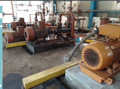
Gambar 5.10 Monitoring Pompa LFO
