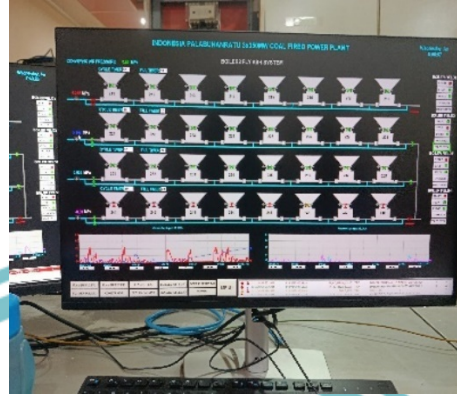
Gambar 5.14 Monitoring Ash Handling Control Room
