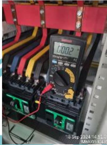
Gambar 4. 8 Test Continuity AC Combiner
