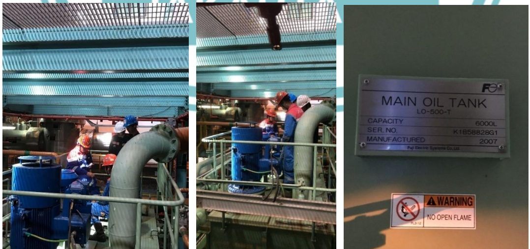
19. Pengambilan Data Main Oil Tank (MOT) Unit 4
